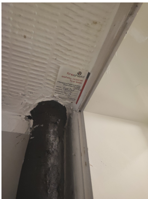
Example fire stopping in common area.
