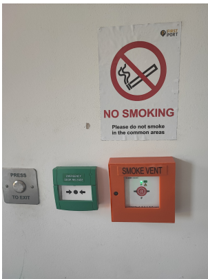
Smoke vent activation point.
